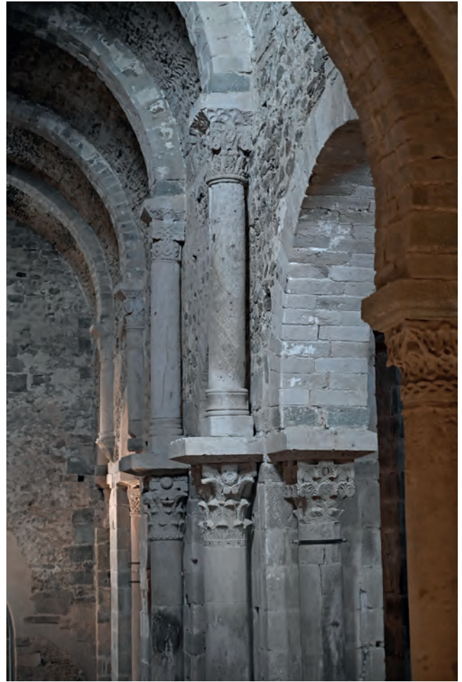
FIGURE 1. Church in Sant Pere de Rodes, second quarter of the eleventh century.
